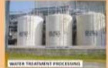
WATER TREATMENT PROCESSING
