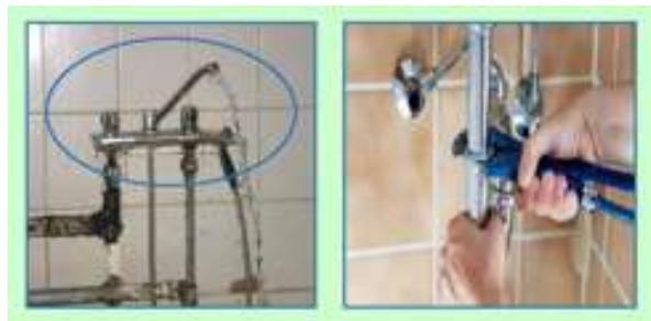
Water Leak upon detection
