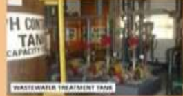
WASTEWATER TREATMENT TANK
